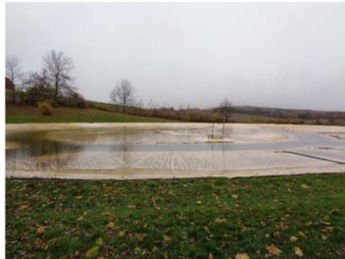
The Palin Hill Reservoir cover protects the City's drinking water from possible sources of contamination, like the accumulated surface water.
